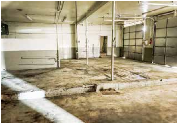
Above: What 2302 Dayton Street looked like when it housed an auto body garage. Right: The inside of the building as it looks today.
