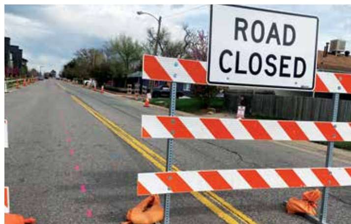
A sign along East 25th Ave. in Northwest Aurora alerts people of roadwork and closures in the area.
